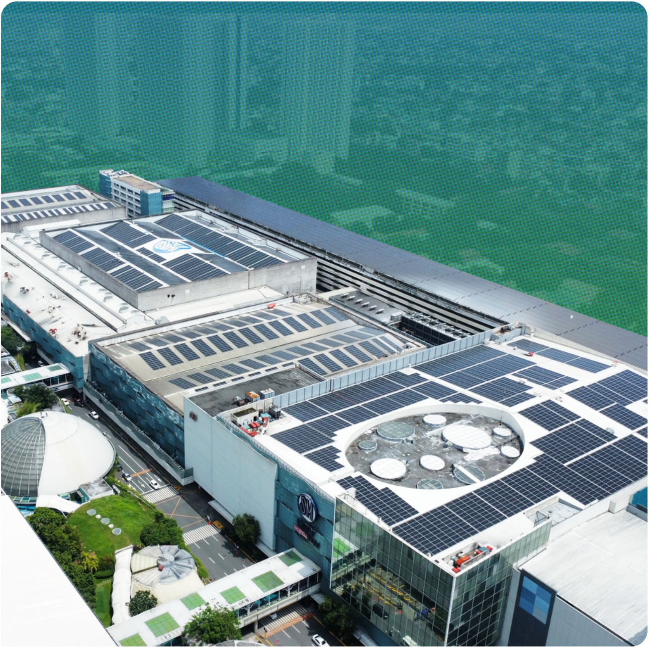
▲ 4.7 MWp ROOFTOP solar photovoltaic (PV) installed at SM North EDSA, the largest rooftop solar on a commercial mall.
